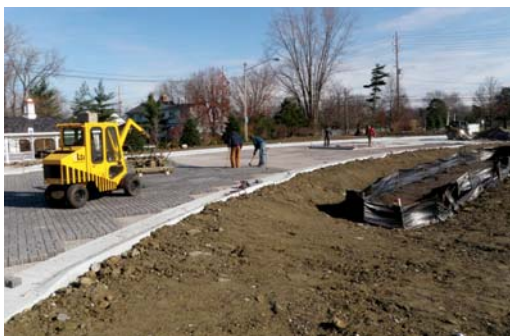
Pervious Paver Underdrain and Curb Cuts Drain to Bioretention Cell
